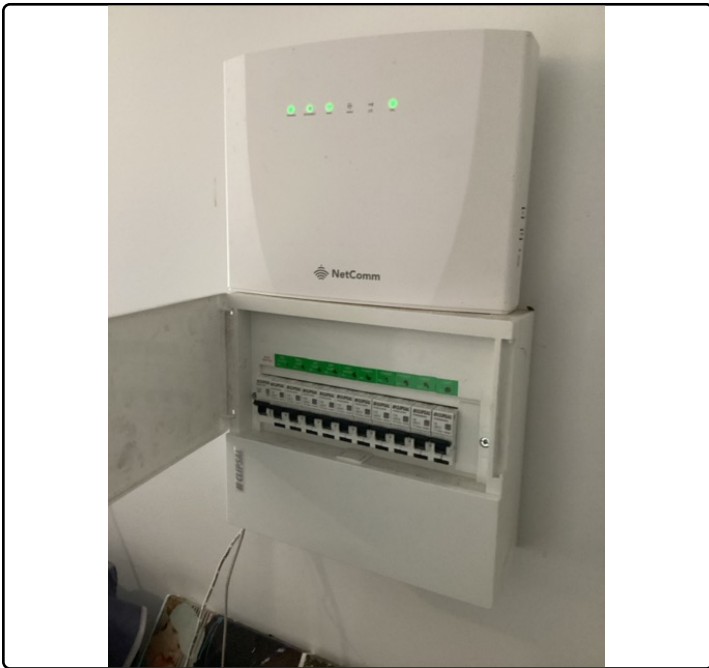
Before Safety switch
