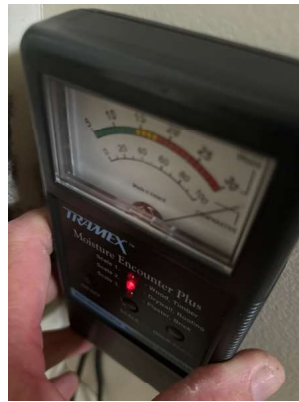
Extremely high moisture behind en-suite in toilet wall
