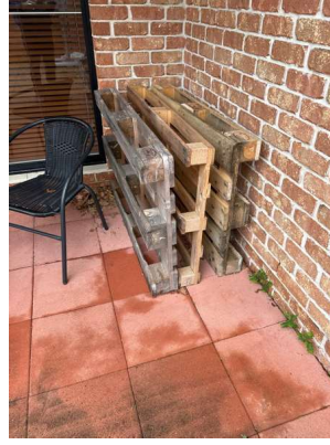
Stored timber against walls
