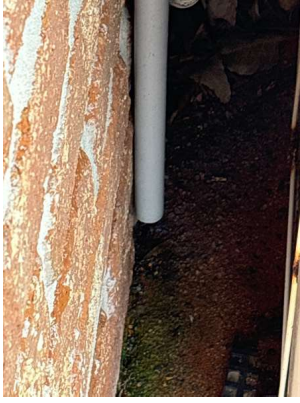
Air con overflow against dwelling
