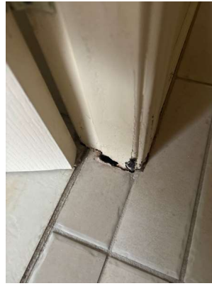
Previous moisture damage in bathroom door frames
