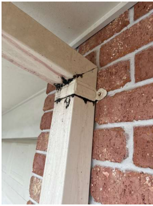
Leaking down pipes
