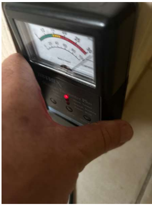
Extremely high moisture in bathroom door frame
