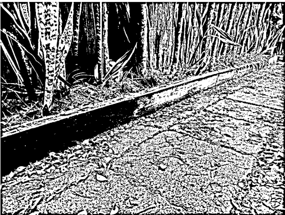
Example of garden edging timbers in ground contact. Would recommend replacing with less susceptible alternatives.
